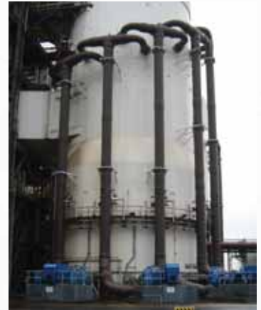
Power Station Absorber
