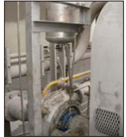
AESSEAL® water management system on slurry pump duty.
