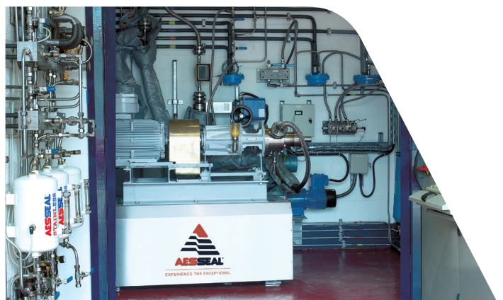
Extensive AESSEAL® test facilities
