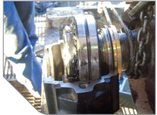
SKF pillow block with LabTecta®66PB in a pulp and paper plant (Case Ref: 3217)
